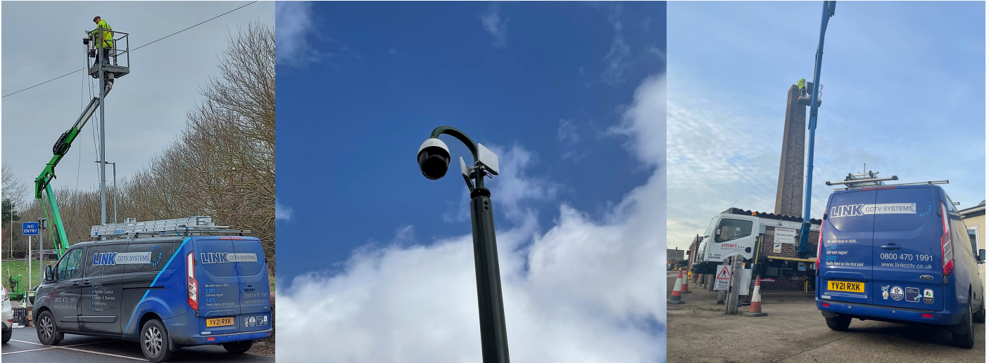
The Link CCTV Systems' Project Team installing wireless repeater transmitters upon a Council building (pictured right).
